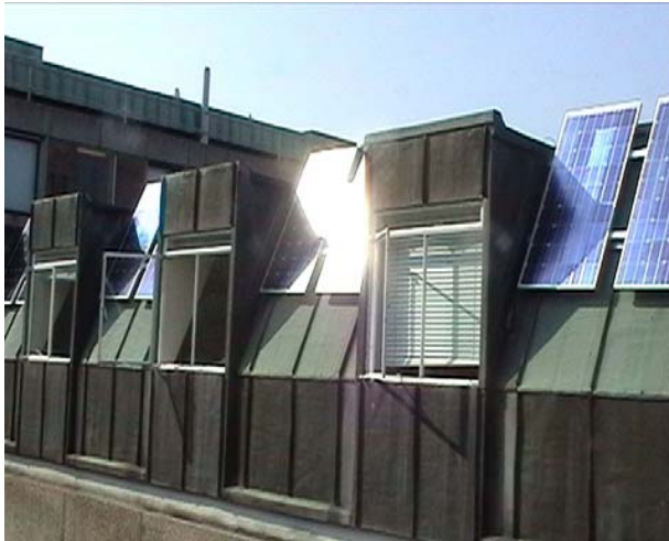
Photo Voltaic panels installed on the roof of the School of Engineering
