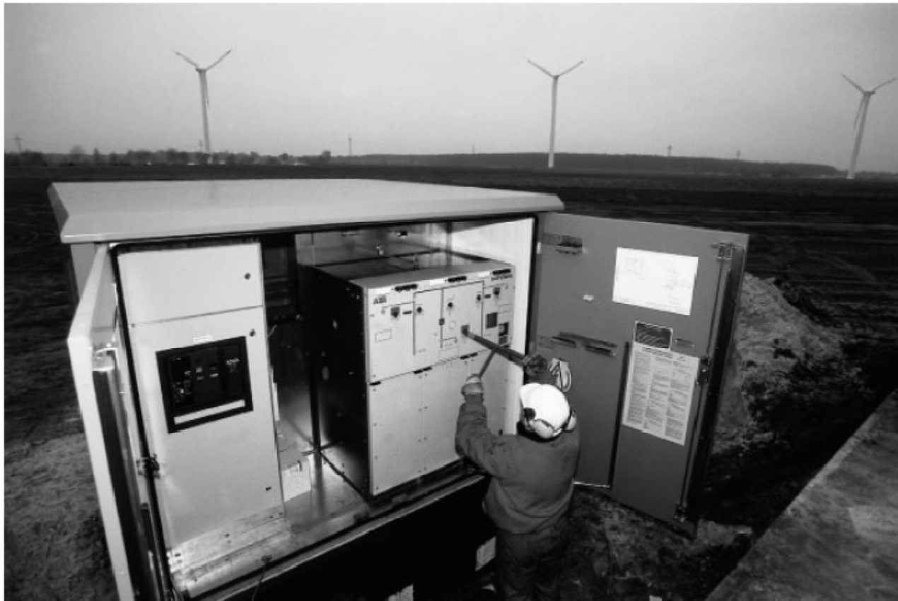
Figure 10.2 Transformer and Switchgear of 1.5 MW Wind Turbine, MV Switchgear on right, LV Switchgear on left (Reproduced by permission of NEG MICON; www.neg-micon.dk )
