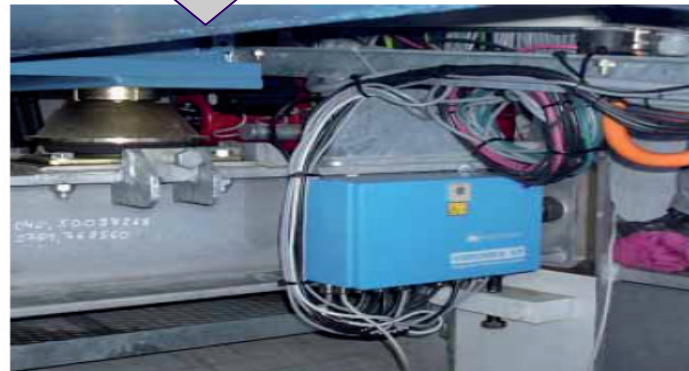
EMC-based installation of a VIBRO-WEB® XP under a 2500 kW generator
